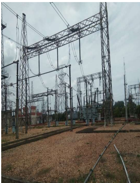
400 kV Durgapur SS
